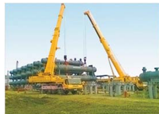
Installation of Heat Exchangers at Compressor Station Yarynskaya under VNM engineers's supervision
